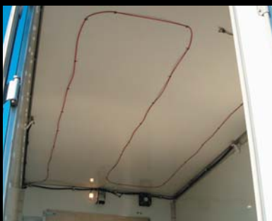
The red Firetrace Detection Tubing is routed from the tank to the shredder truck's grinding and collection areas, ensuring that detection is close at hand in the event of a fire.
